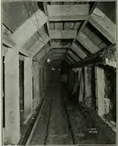
Interior of Tunnel Showing Timbering Spaced to Allow Rock to Be Removed as It Swells. (Photo by Geo. F. Fanning.)
